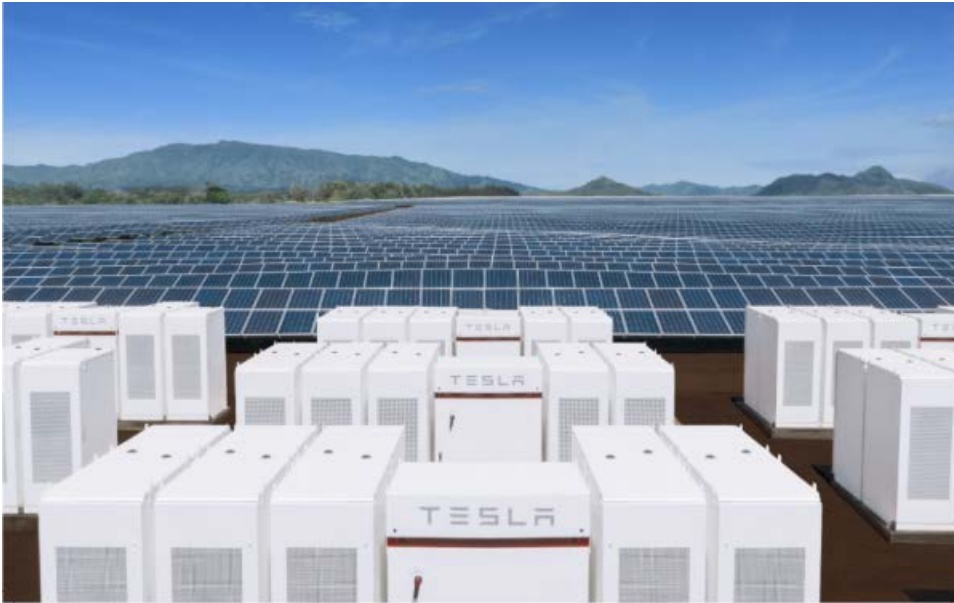
Figure 2. Example of a Powerpack Site
